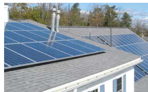
Leicester Police Station – 22.40 kW PV system
