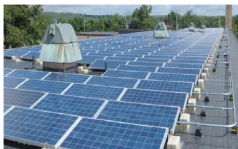
Leicester Memorial School – 90.72 kW PV system
