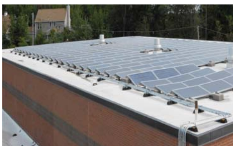
Leicester High School – 172.42 kW PV system
